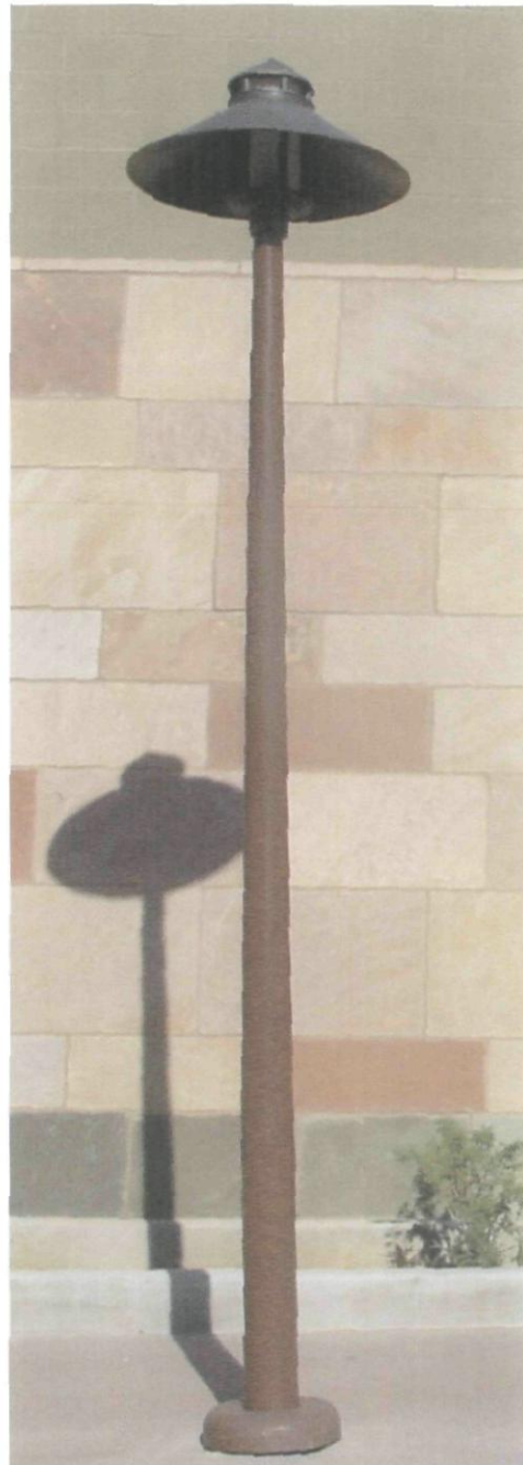
Pole Mounted Area Lighting (Max - 12' Ht.)
