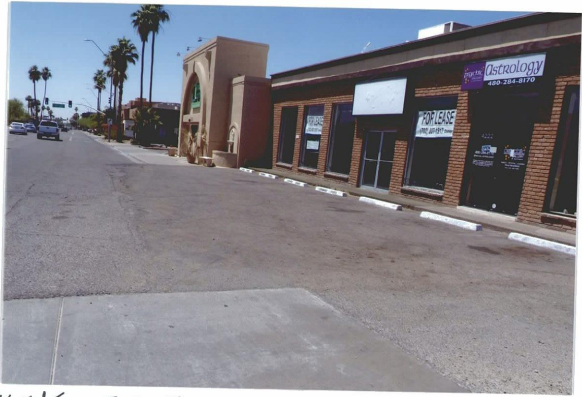
LOOKING SOUTH DRIVEWAY ENDS PATCHWORK ASPHALT UNDEFINED WALK'
