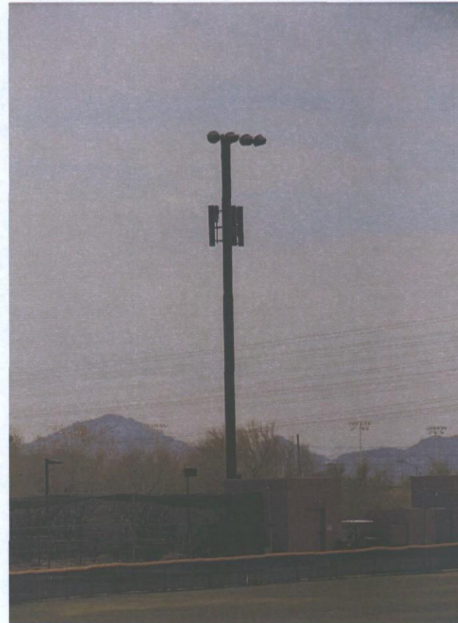
REPLACEMENT OF EXISTING ANTENNAS WITH NEW ANTENNAS. ADDITION OF J-BOX AND THREE (3) RRU'S: 1 RRU PER SECTOR.
