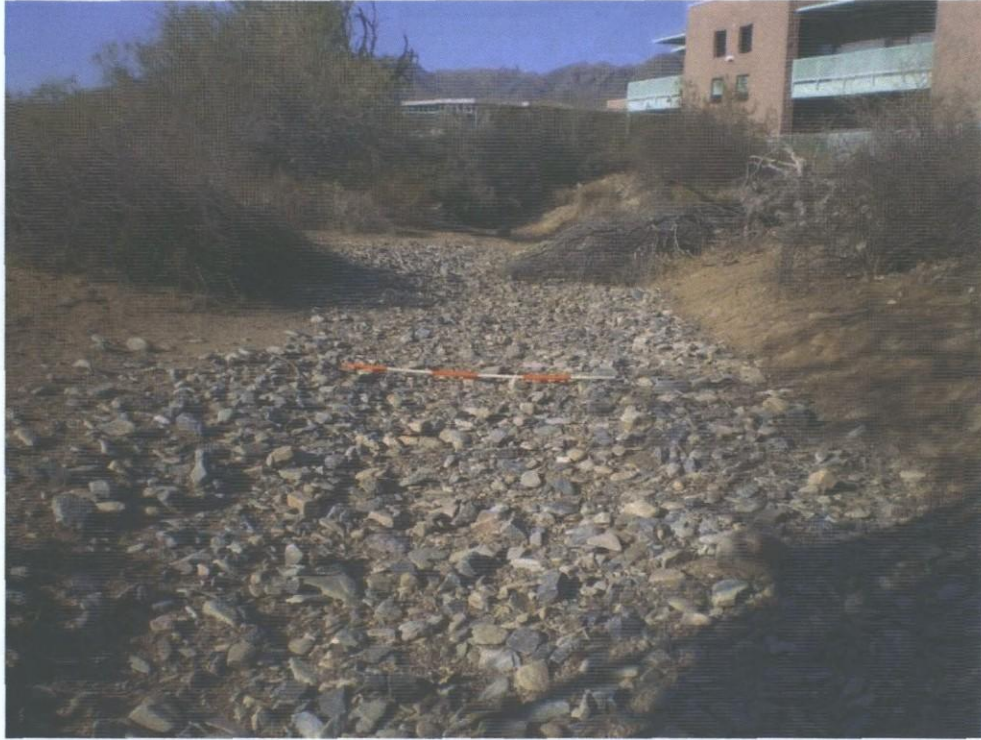
Photo 33. Upstream view of drainage west of 98 th Street (school on east side) (10 ft)
