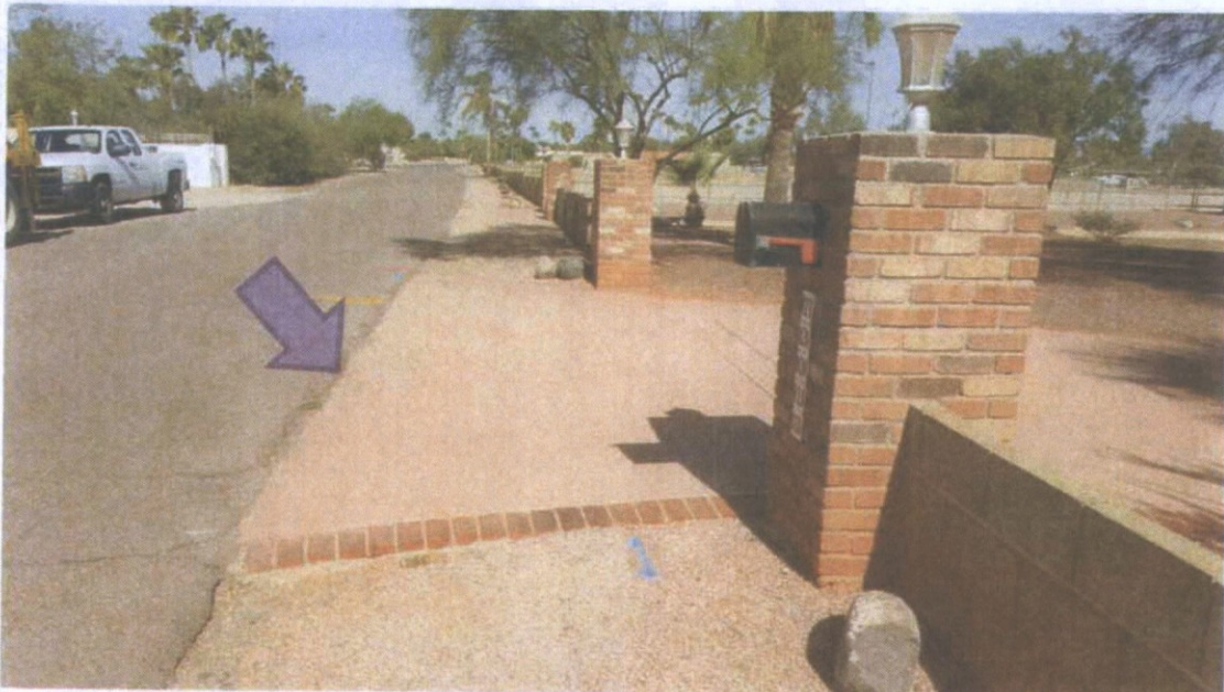
Looking north at the location of A-1 and C-1. Note the lip at the junction between the asphalt and concrete.
