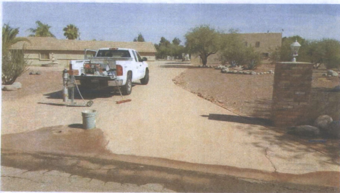
Coring operation at C-2. Stress cracking at the entrance corner on the concrete. Excessive alligator cracking in the asphalt as it abuts the concrete.
