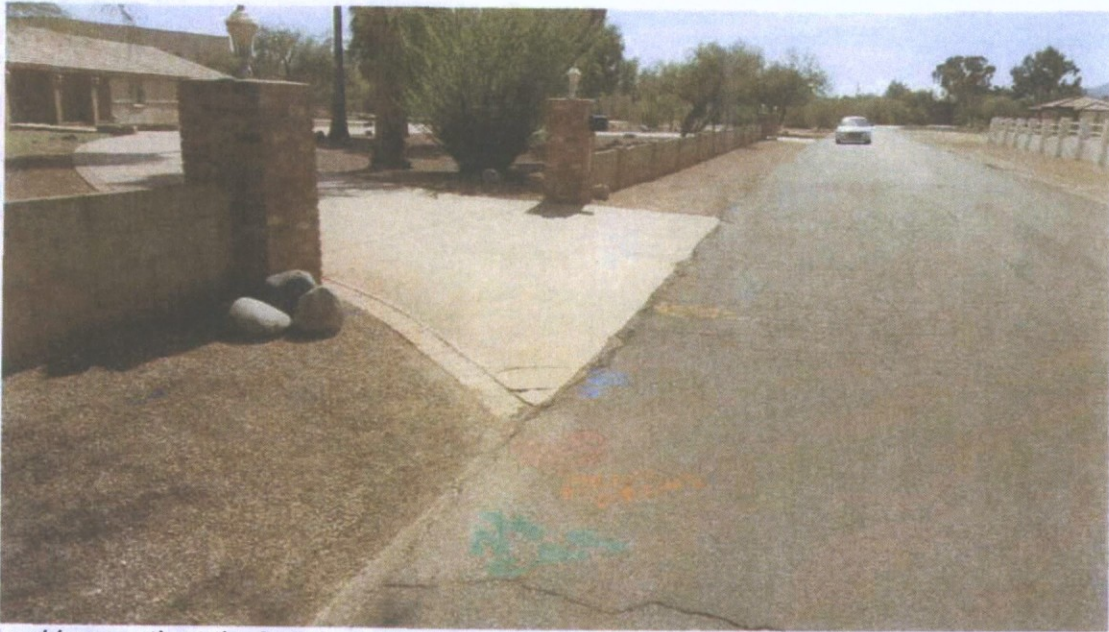
Looking south at the locations of A1 and C-1. Note the excessive alligator cracking, which typically suggests a lack in subgrade support, water infiltration, inadequate asphalt cement content in the asphalt mixture, or inadequate thickness design for the soil conditions.
