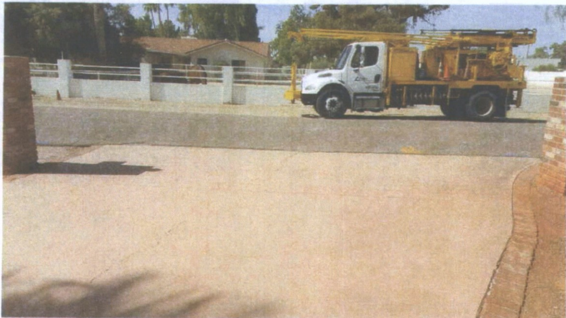
Looking west at the locations of A-1 and C-1. Note the presence of longitudinal and transverse cracks in the concrete, typically indicating either soil expansion or the lack of control joints.
