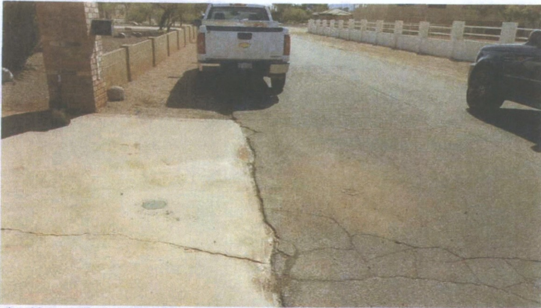
Looking south at the location of A-2 and C-2. Separated locations of alligator cracking.
