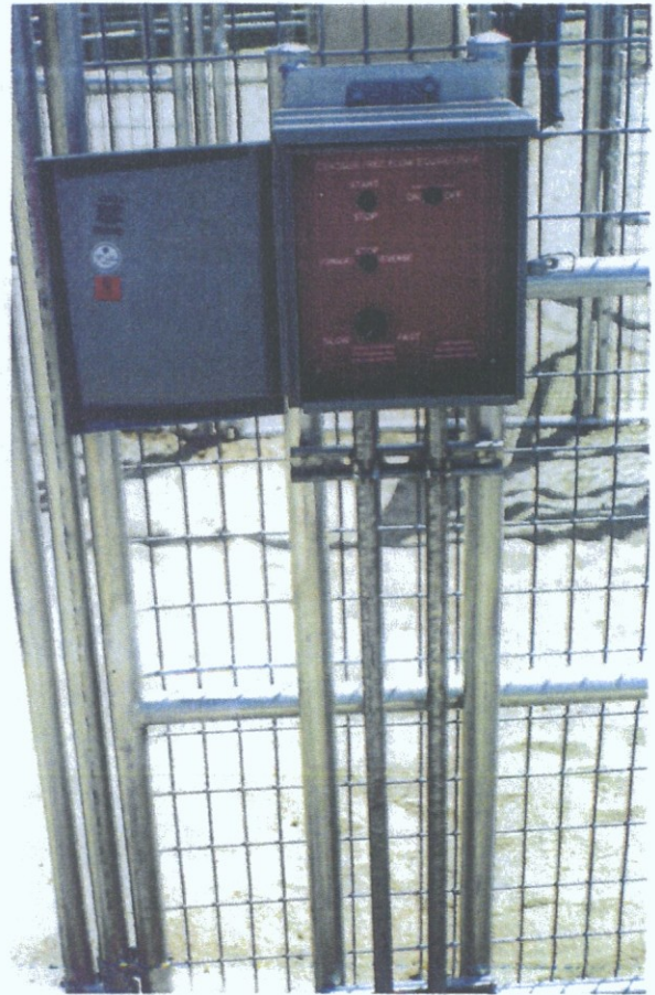
Control Box with individual controls for: Start/Stop, Screen Shocker On/Off, Forward/Reverse, and Adjustable Speed Control
