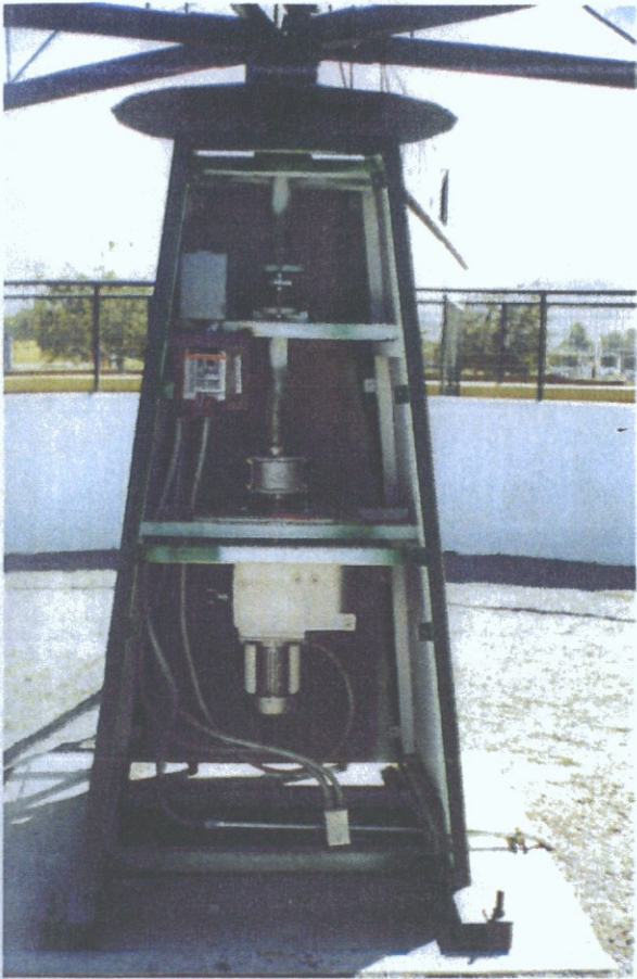
Interior view showing: Motor, Gearbox, Falk Coupling & Computerized Controller.
