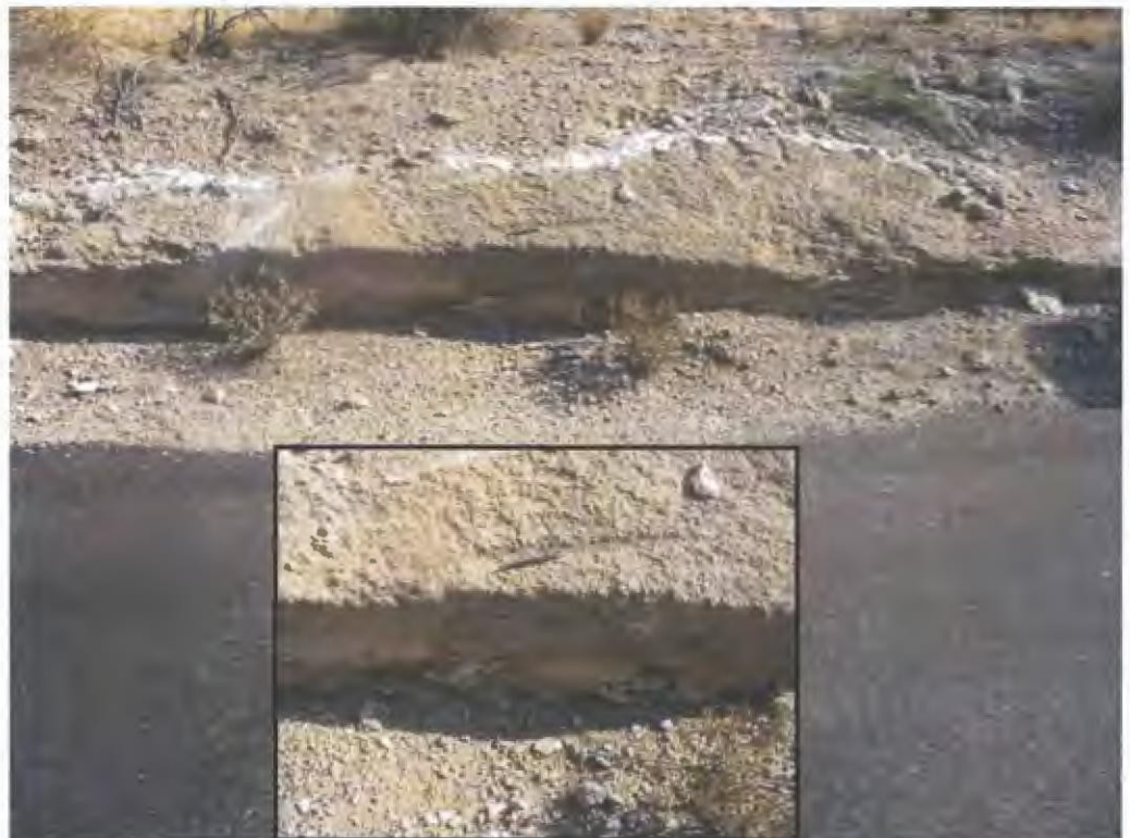
Figure 22; Photo 2: Exposed section of well-formed Stage IV-V caliche locally capping the underlying decomposed granite and less weathered granite at depth. Outcrop exposed in shallow road cut paralleling the north side of Black Mountain Road near seismic survey line BM -S6.
