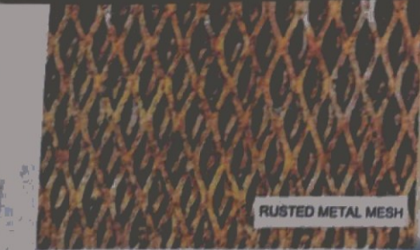
C1 SMOOTH STEEL RUSTED & SEALED
