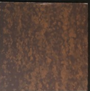
3 RUSTED STEEL western stakes metal
