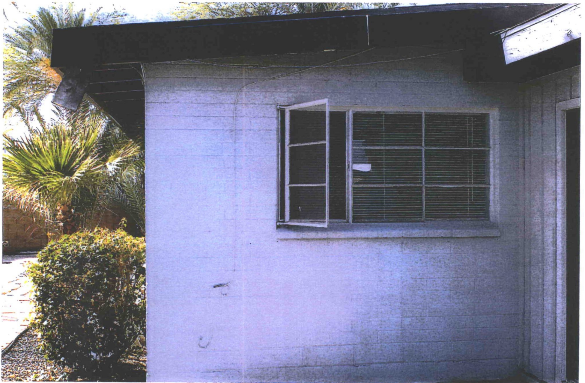
Deterioration of fascia board. Back of property.
