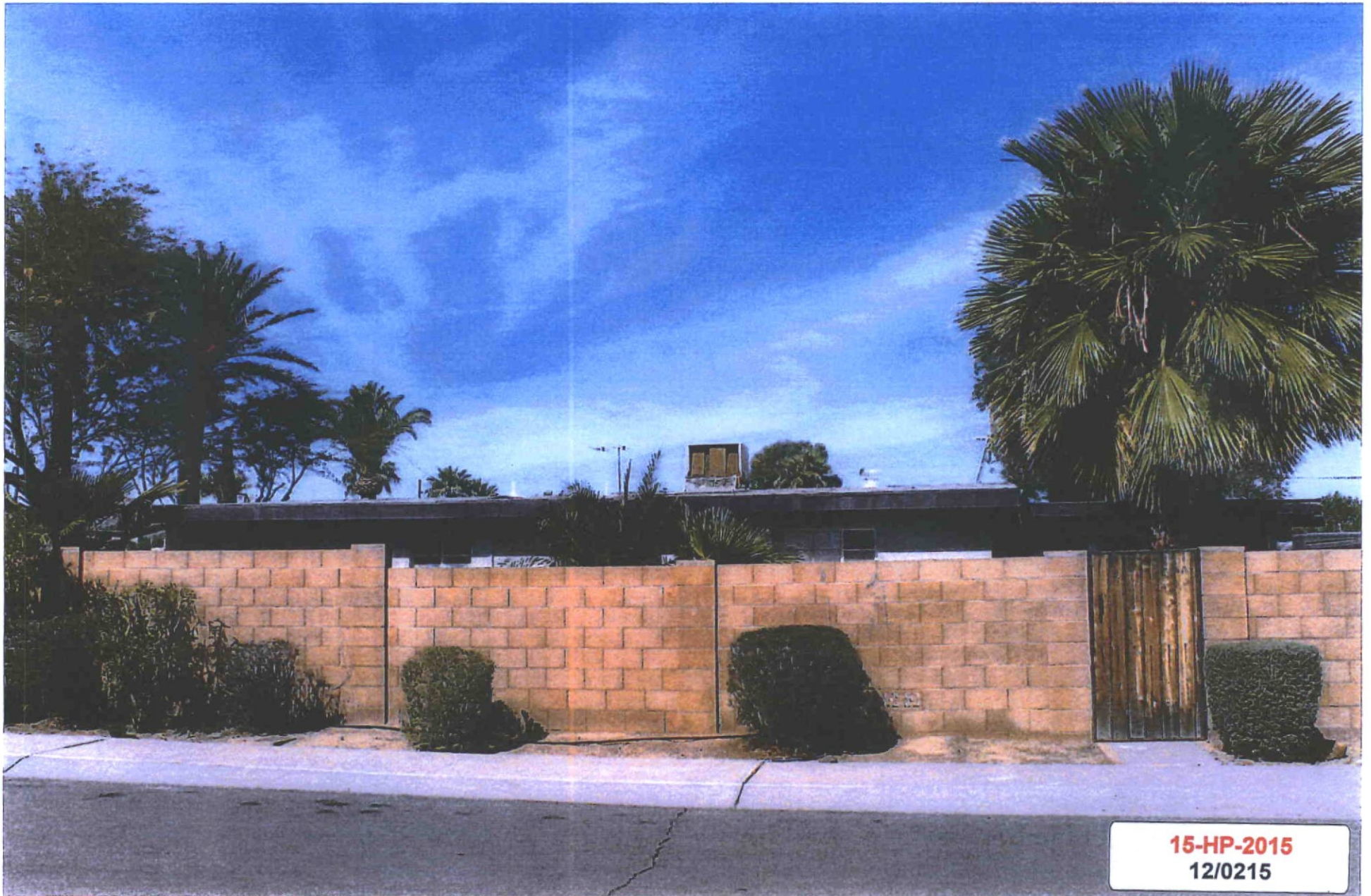
Side view of property, from Monte Vista. Project will remove deteriorated swamp Corder.
