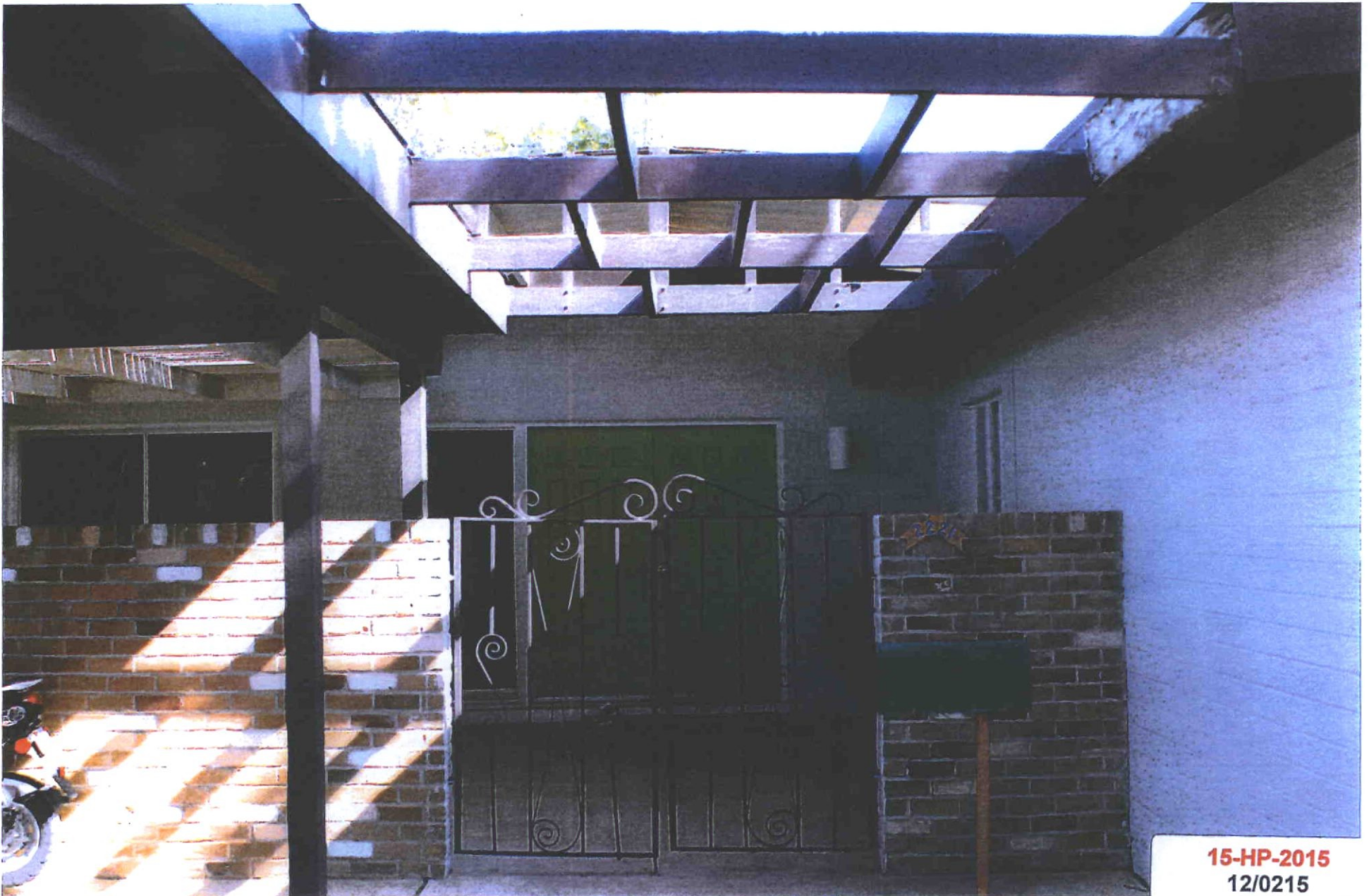
Open pergola and entry way, visible from 72nd Place. Picture shows deteriorated wood.
