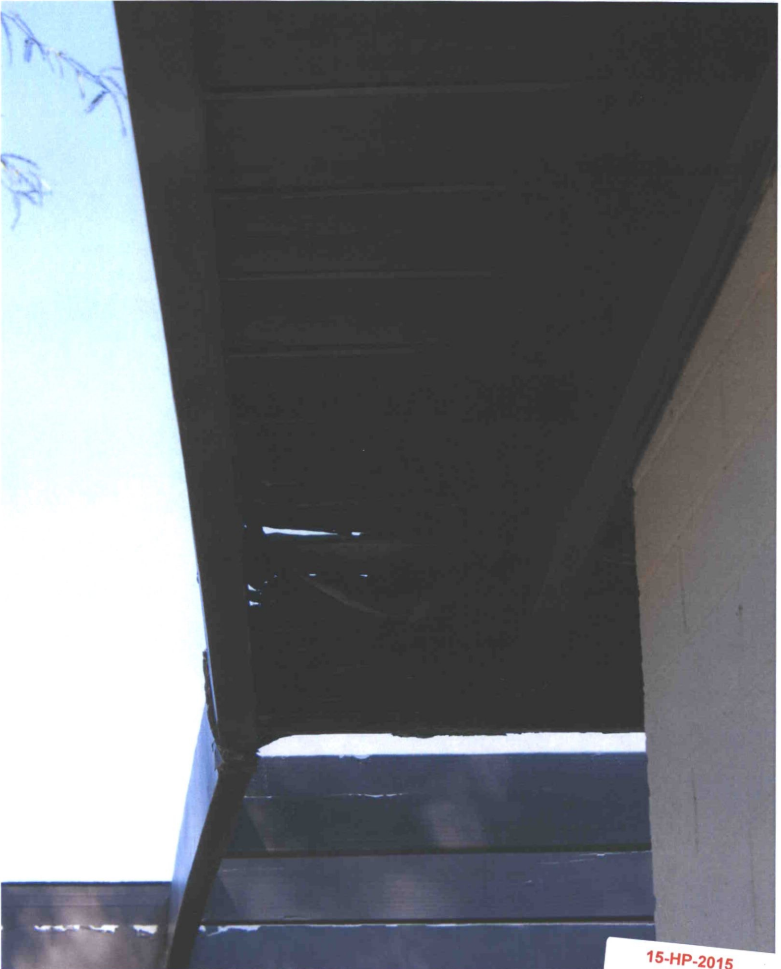
Damage: tongue + groove, fascia board
