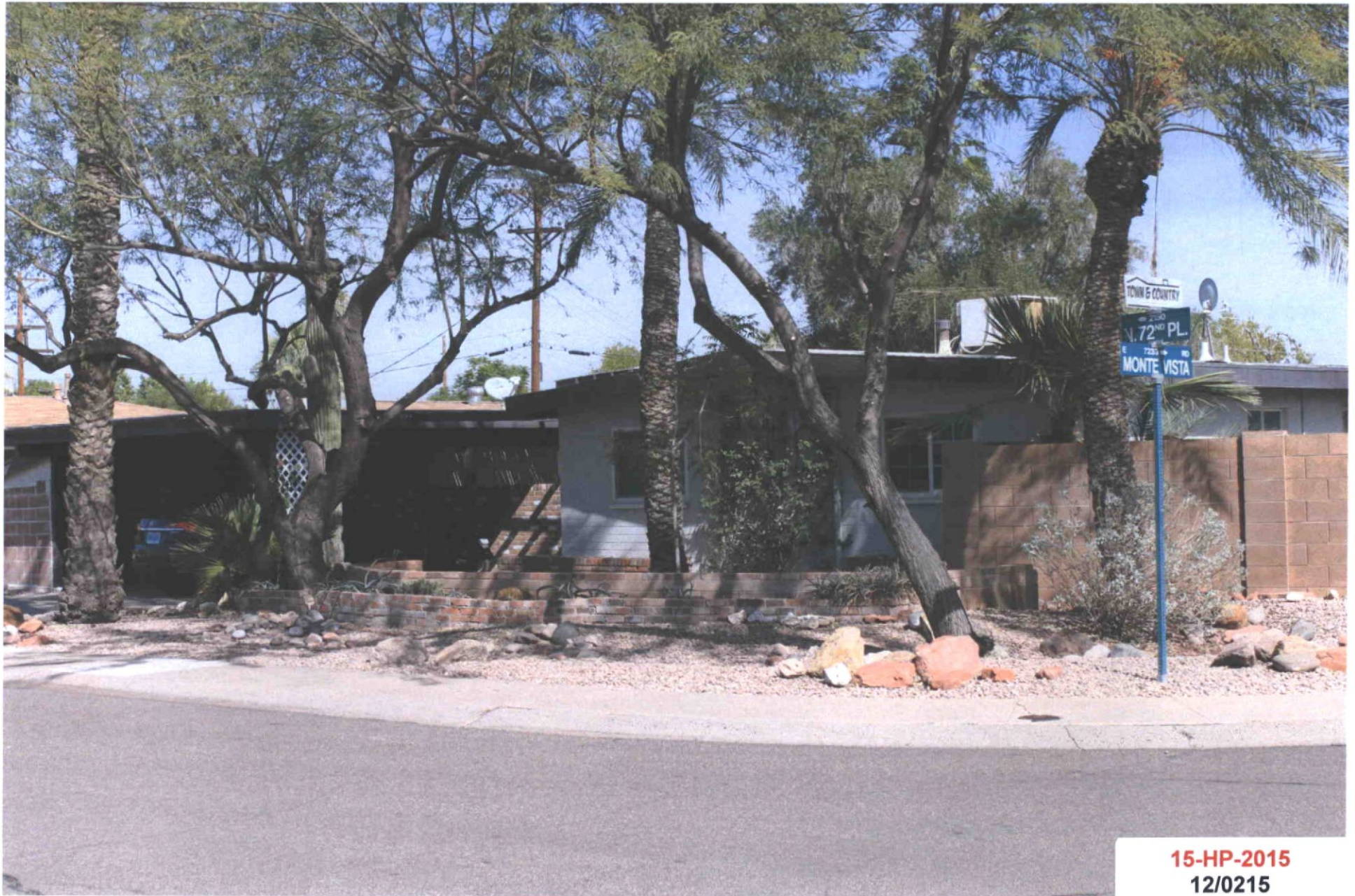
Picture from 72nd Place & Monte Vista. Deteriorated Swamp cooler and old antennas will be removed as part of the project.
