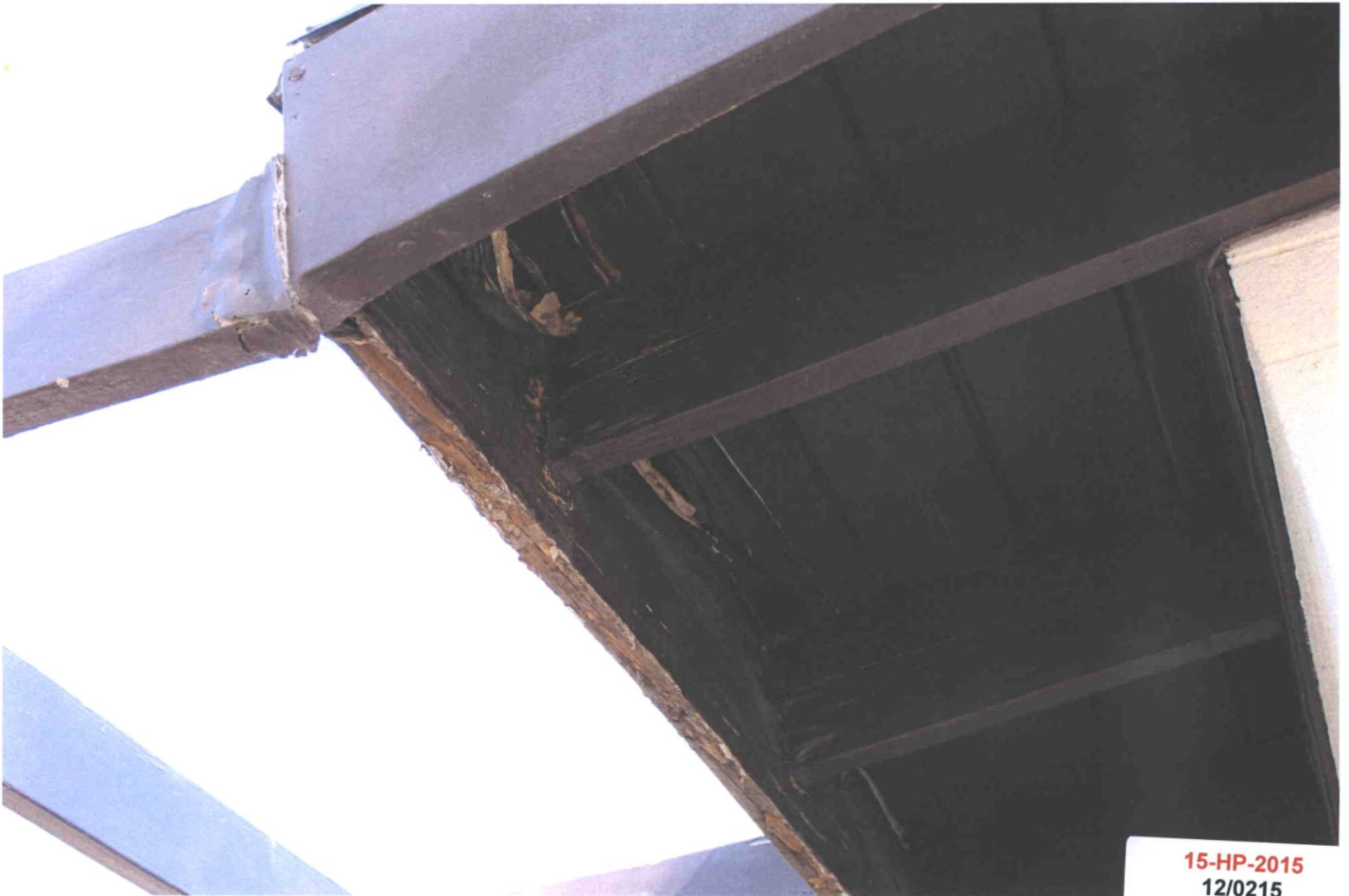
Picture of deteriorated: wood, trim, tongue and groove, fascia and pergola.
