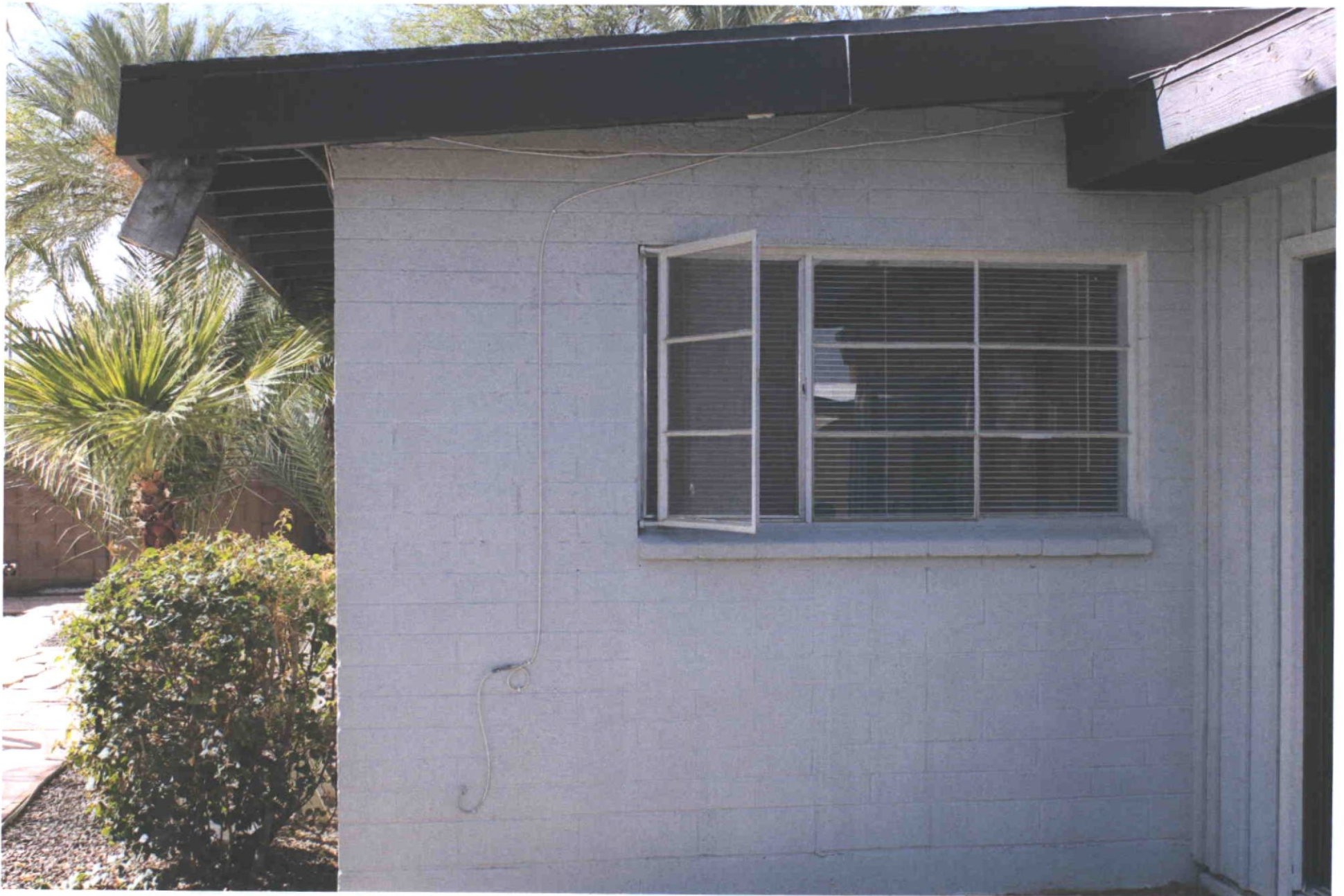
Deterioration of fascia board. Back of property.
