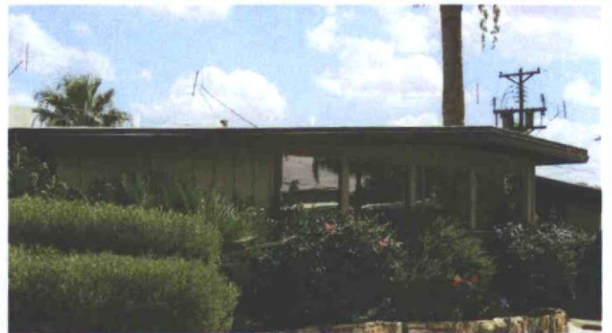
The board and batten siding and window-band are original elements. Use of wood on the upper half of the house was comparatively rare. All examples of wood siding are therefore important to retain.
