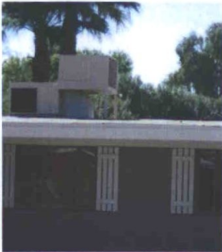
Roof mounted mechanical units have a major impact on the appearance of the house.
