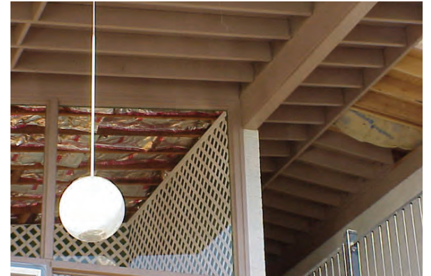
Construction photos from the roof and balcony repairs of 2000 disclose no clues of connectors.
