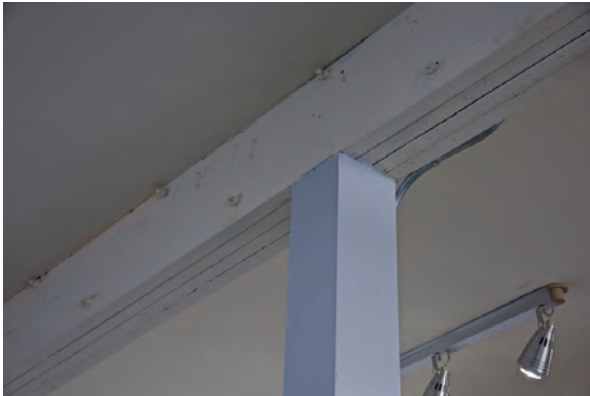
Surprisingly, the beam connections at posts and walls have no visible metal connectors.
