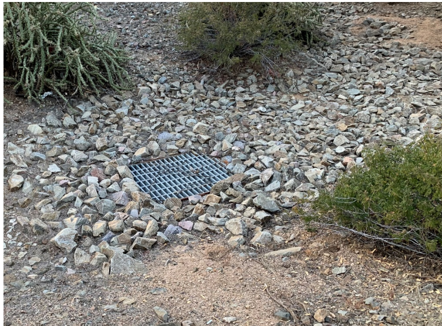
Figure 5. Typical Grate Inlet along 60-in Storm Drain
