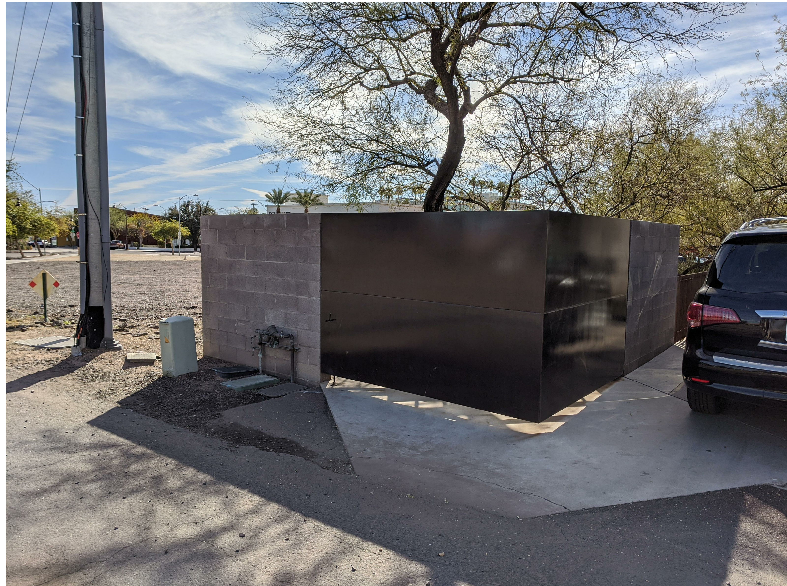
22 VIEW LOOKING TOWARDS THE SOUTHEAST FROM THE ALLEY AT THE EXISTING WASTE ENCLOSURE
