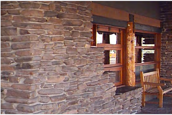
ENCOURAGED - Use of materials with coarse texture and colors associated with the desert southwest further define Old Town's sense of place.
