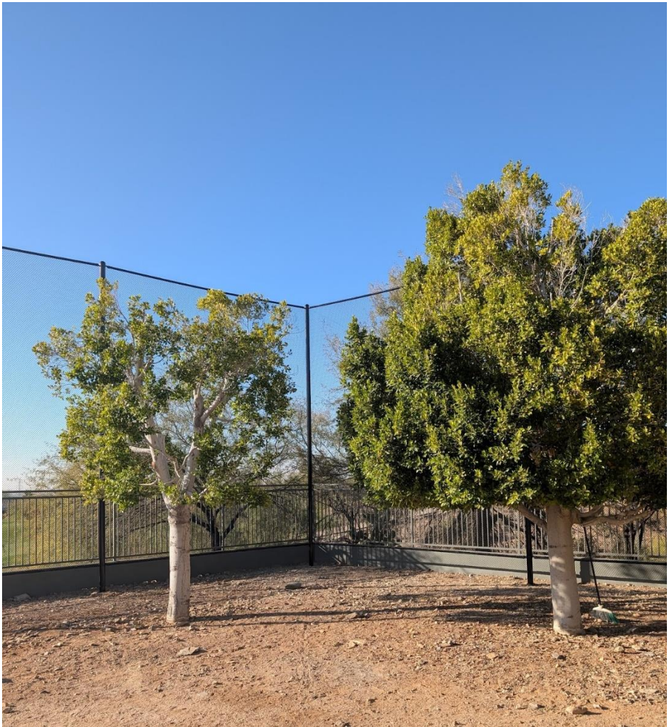
Current installation – 20 feet
