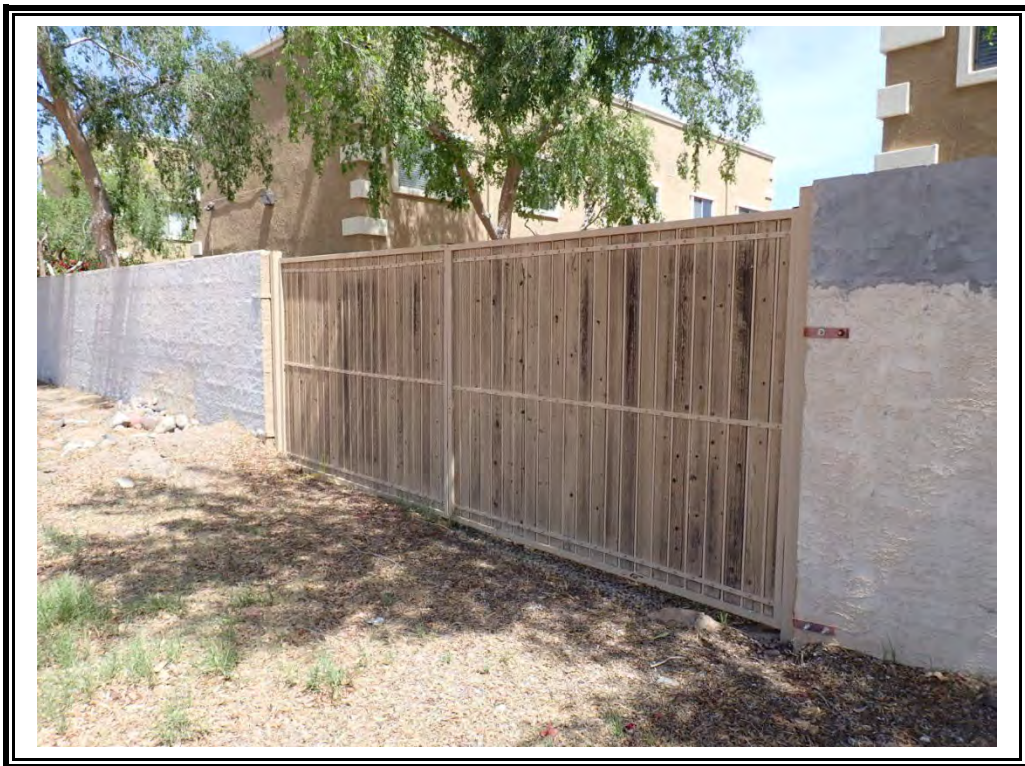
View of gate on Polk Street at the center east side of the subject parcel grouping
