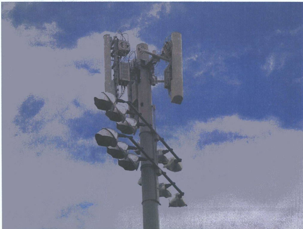
Existing antenna array
