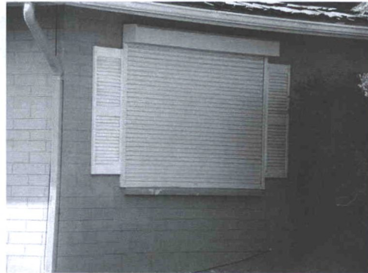
Rolling steel shutters adversely affect the character of the original windows.
