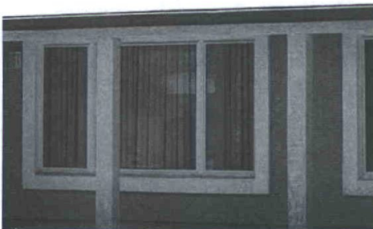
These replacement windows do not match the original. There are no through-the-glass muntins between smaller panes of glass like the original window pattern.
