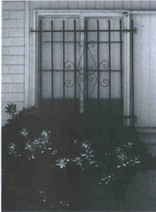
Metal security grilles detract from the original appearance of the windows and inappropriately cover both the boxed window and reveal in this example.
