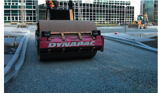
Aggregate base and subbase are spread and compacted; pavers are delivered ready to install. After placement, joints and/or openings are filled with small aggregate. Then pavers are compacted.
