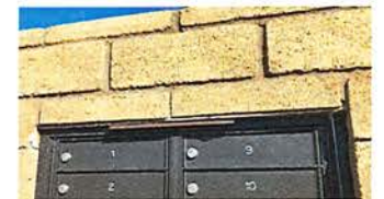
DOWN LED LIGHT AT MAILBOX MANUFACTURER: ALLIANCE OUTDOOR LIGHTING MODEL #: SL85-LED
