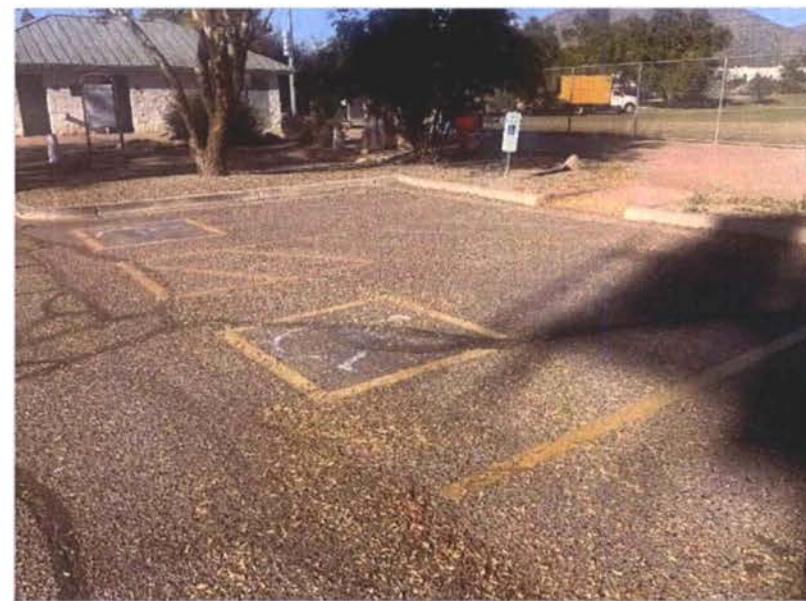
Figure 7: Fading Accessible Parking Spot Paint
