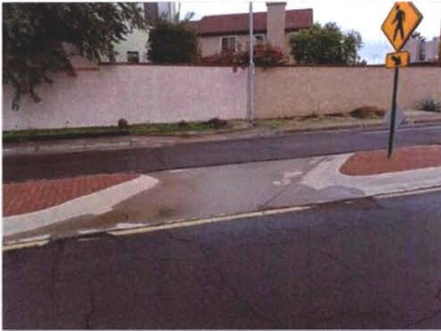
Figure 16: Median Refuge Island with Missing DWS
