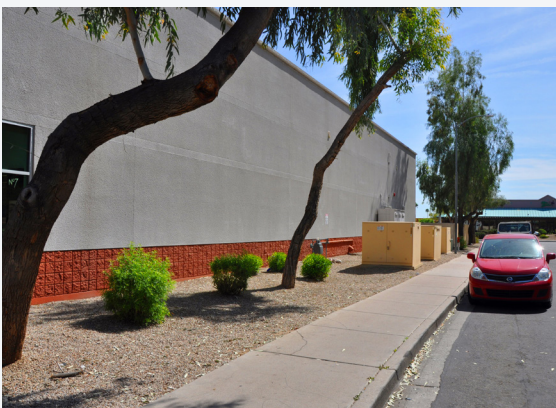
DISCOURAGED - Unscreened electrical equipment and blank building wall is highly discouraged, particularly facing a public street.
