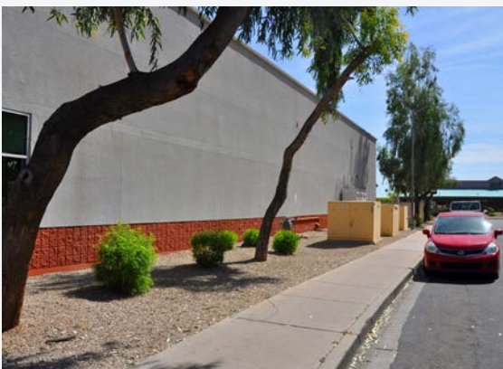
DISCOURAGED - Unscreened electrical equipment and blank building wall is highly discouraged, particularly facing a public street.
