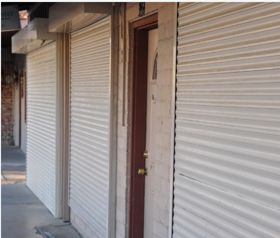
DISCOURAGED - Exterior mounted, roll-down, security doors on street-facing storefronts.
