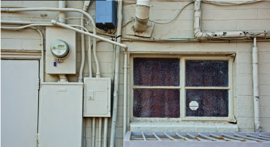
many generations of electrical system modifications are evident on the rear elevation
